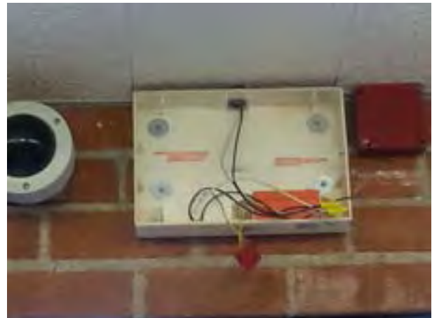
Disabled fire alarm sign with exposed wires
